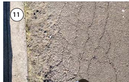
11 Pavement and concrete sections around school need repair.
